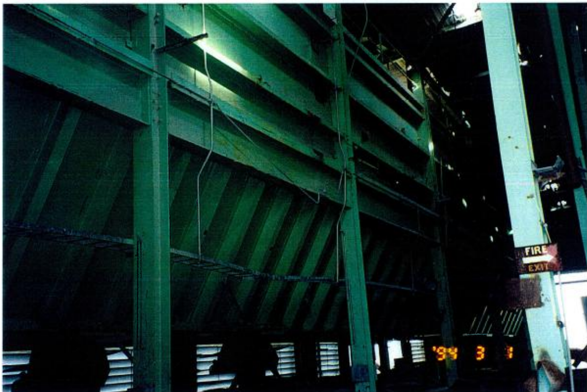
One of three large hoppers on the 7th and 8th floors, containing asbestos material.
