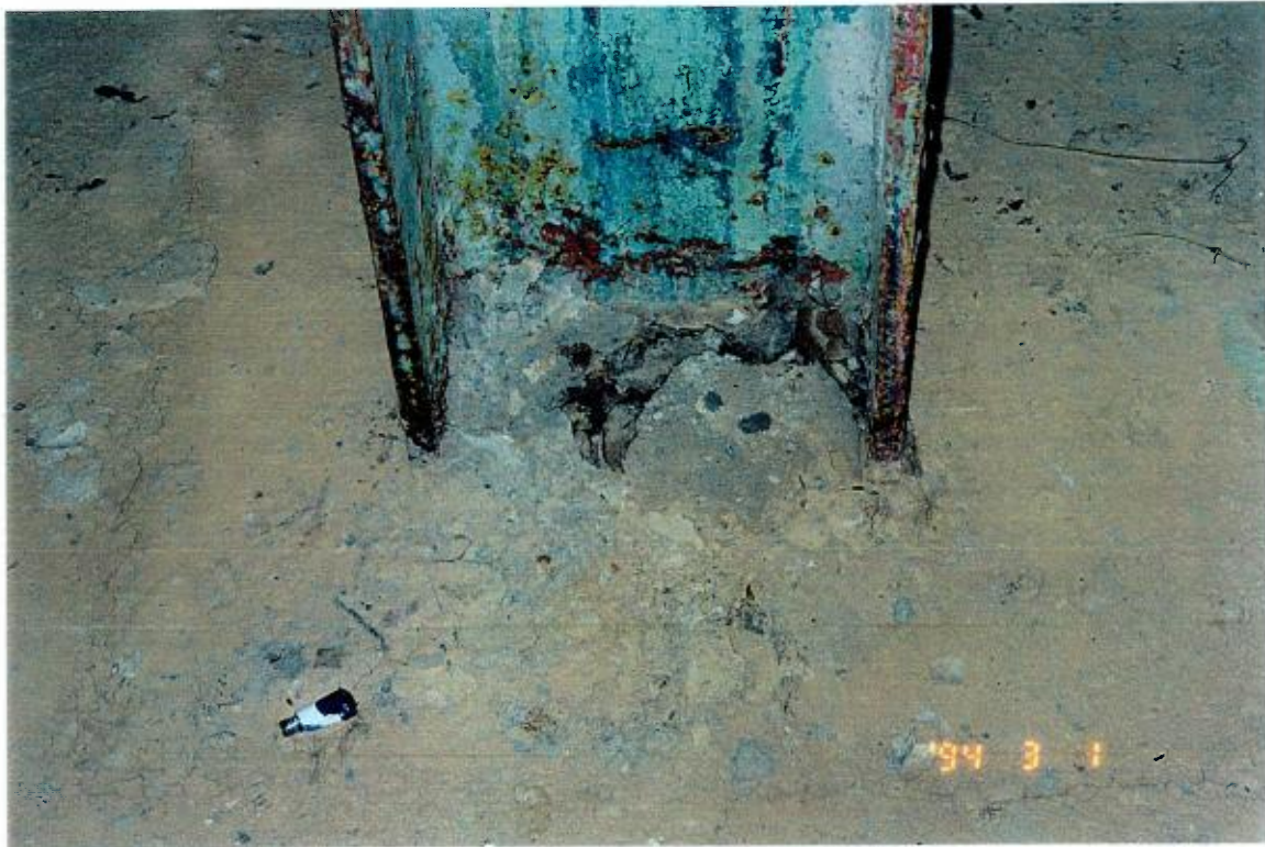
Asbestos fibre on the floor around structural columns.
